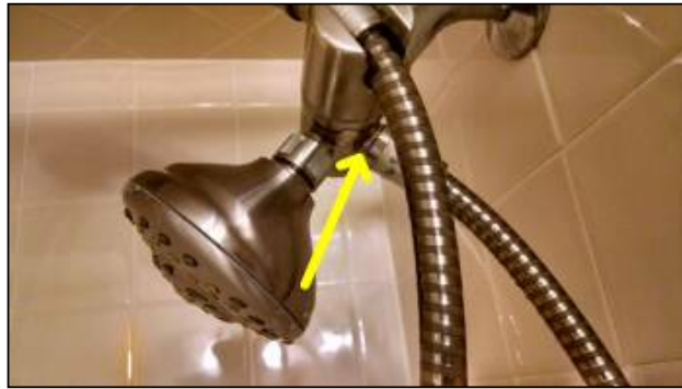
Leaking shower head
