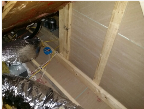
Areas missing insulation
