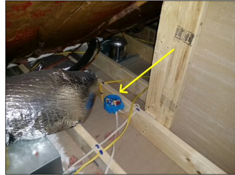
Junction boxes should have covers
