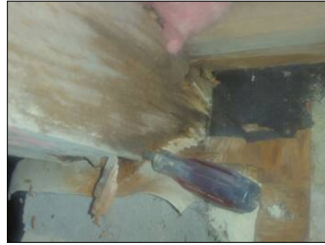
Wood damage due to biogrowth
