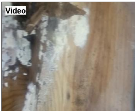
CLICK to view VIDEO - example of damage below doors
