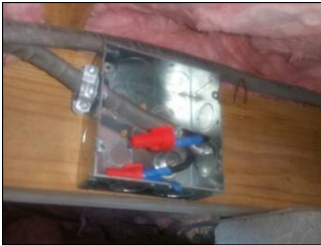
Junction boxes should have covers
