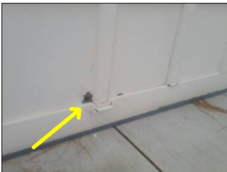
Damage at garage door
