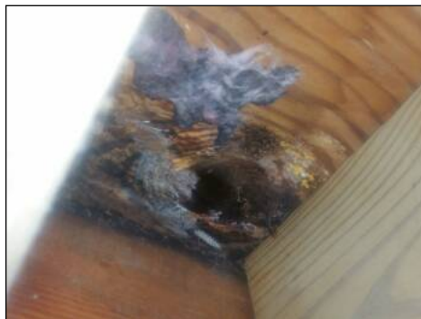
Elevated moisture observed
