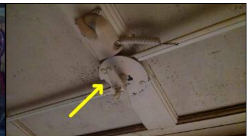
Manual lock installed with opener present
