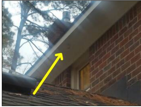
FYI: Auxiliary condensate drain location
