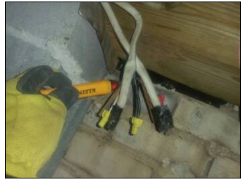
Wiring should be in a junction box
