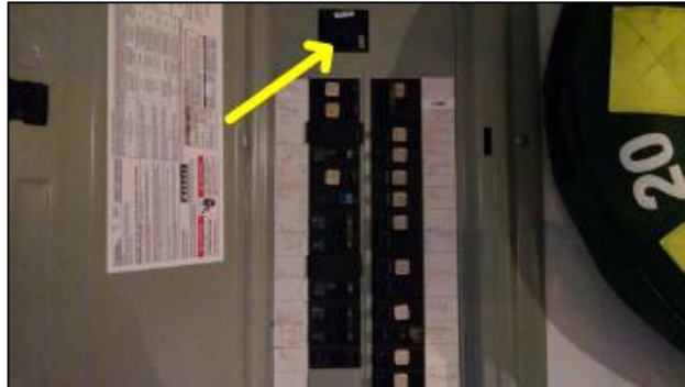
Main disconnect - garage
