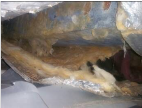
Insulation damaged at ductwork
