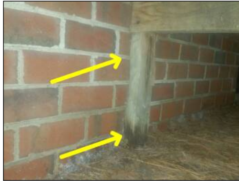
Recommend adding additional support for girders
