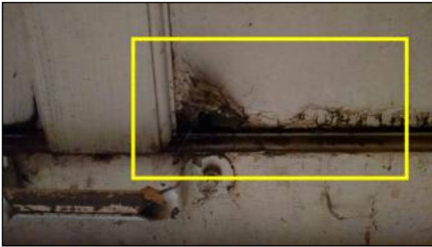
Moisture damage at door
