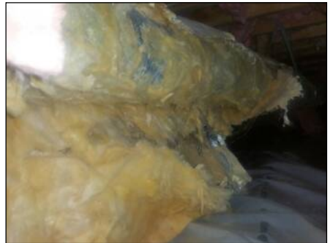
Insulation damaged at ductwork
