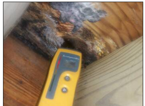
Elevated moisture observed
