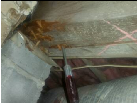
Damage at beam(s)
