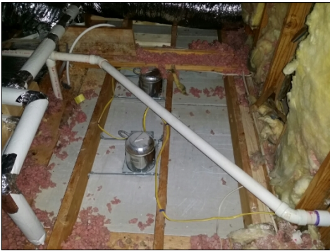
Areas missing insulation
