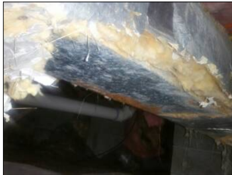
Insulation damaged at ductwork
