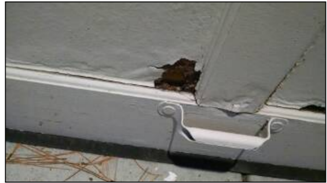
Moisture damage at door
