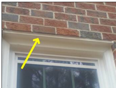
No weep holes at sealant
