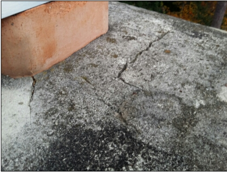
Chimney crown cracking
