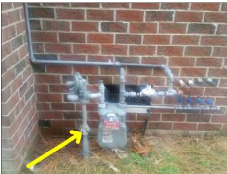
Main Gas shutoff
